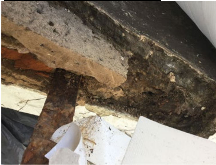
Close Up of Remains of Balcony Structure
